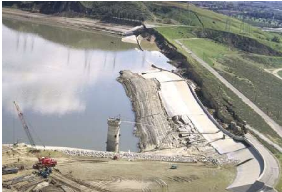
Figure 12. Lower San Fernando dam after earthquake of 9 February, 1971. ( Source: Earthquake Engineering Research Center, University of California, Berkeley )
