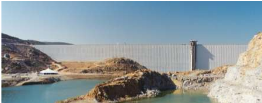
Figure 11. Exposed PVC geomembrane at Olivenhain Dam (courtesy Carpi Tech )
