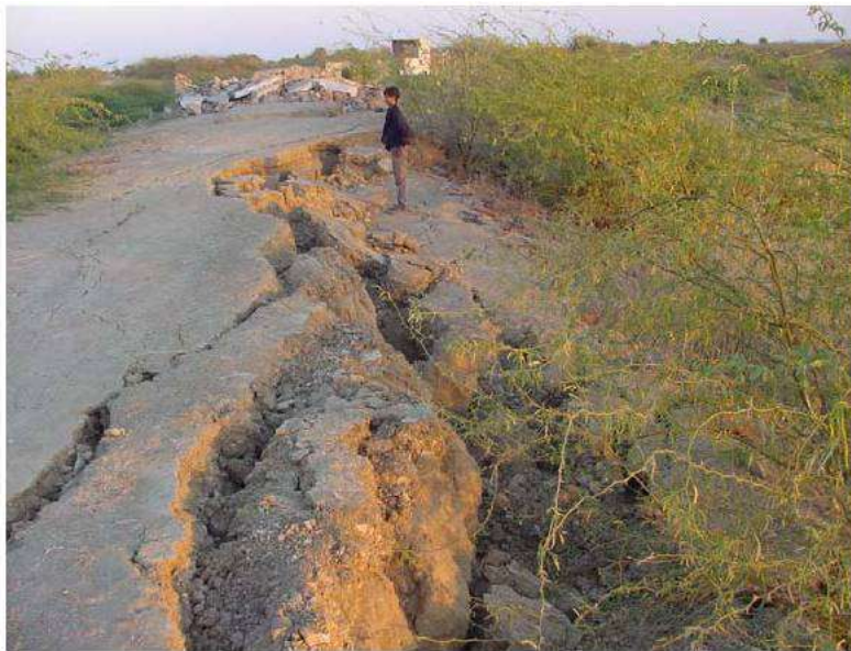
Figure 7. Damage in Bhuj earthquake of 26 January, 2001 ( Courtesy Prof S.K.Jain )
