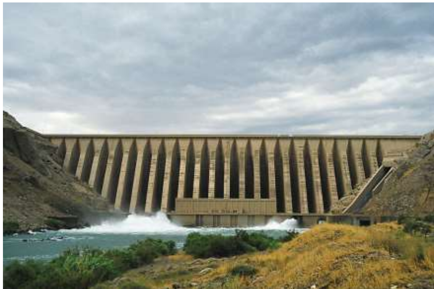
Fig. 6. Sefid Rud buttress dam was damaged near the crest due to ground shaking during the magnitude 7.5 Manjil earthquake of June 20, 1990.
