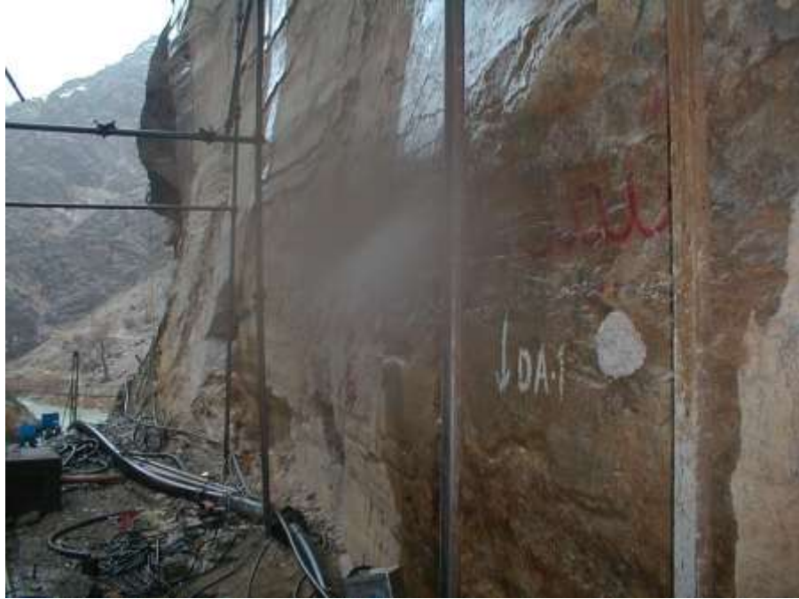
Figure 14. Secondary fault at left abutment of Rudbar-Lorestan dam in Iran
