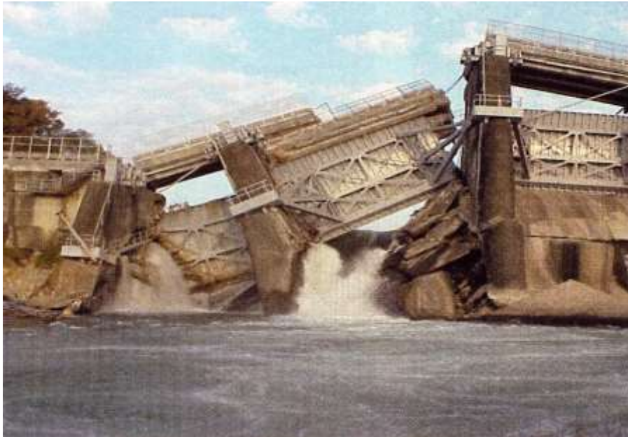
Figure 13. Shih-Kang dam after the earthquake of 21 September 1999.
